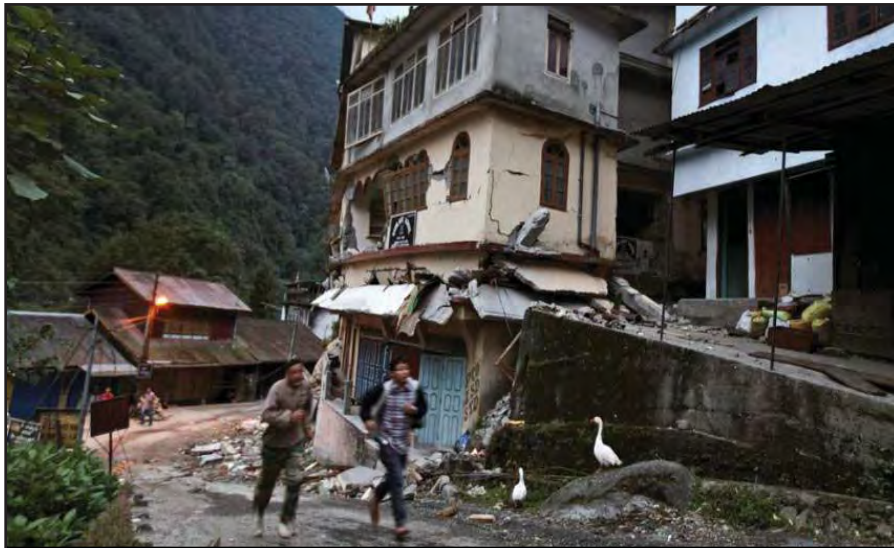
Earthquake survivors run past a school building in Chungthang, damaged in the 2011 Sikkim earthquake
